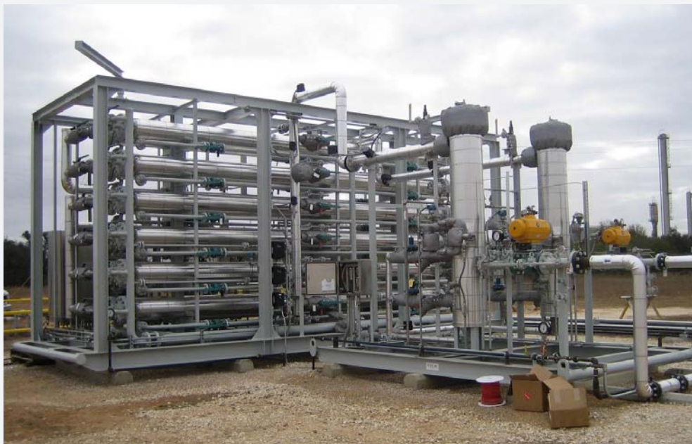
MTR supplied CO 2 removal system operating at a Texas gas well
