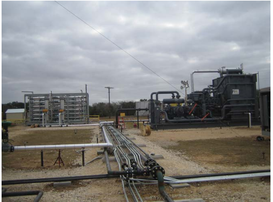
A CO 2 removal unit installed at a wellhead site
