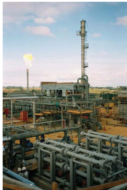
Gas turbine power station with fuel gas conditioning unit
