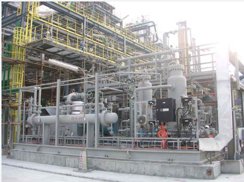
This propylene/nitrogen recovery unit was recently started up in Asia.
