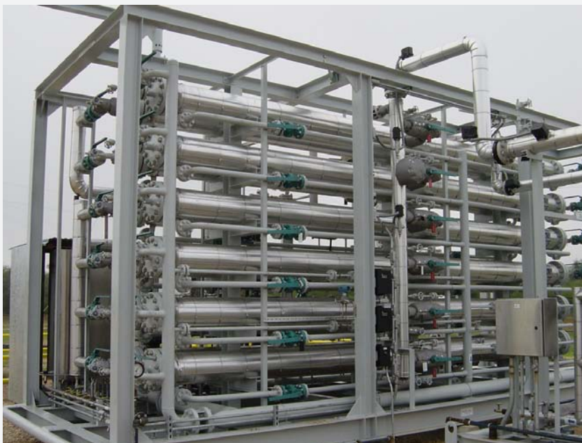
Skid mounted CO 2 removal system
