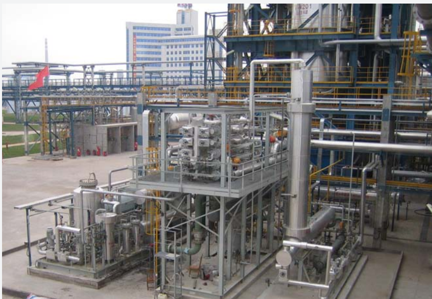
This VaporSep® unit recovers hydrocarbons from offgas
