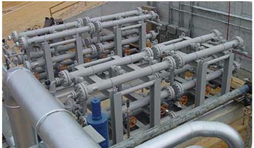
Membrane skid for hydrocarbon recovery
