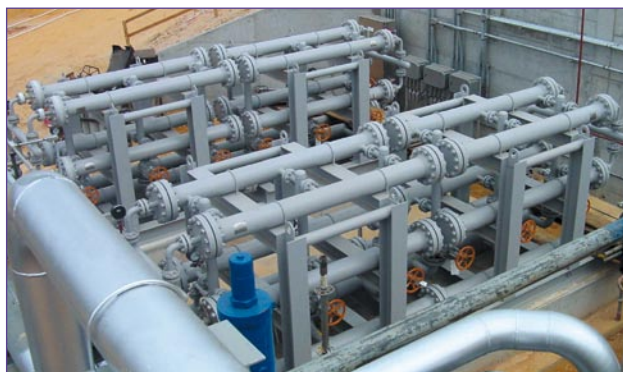
Figure 4. Membrane skid with spiral wound modules.
