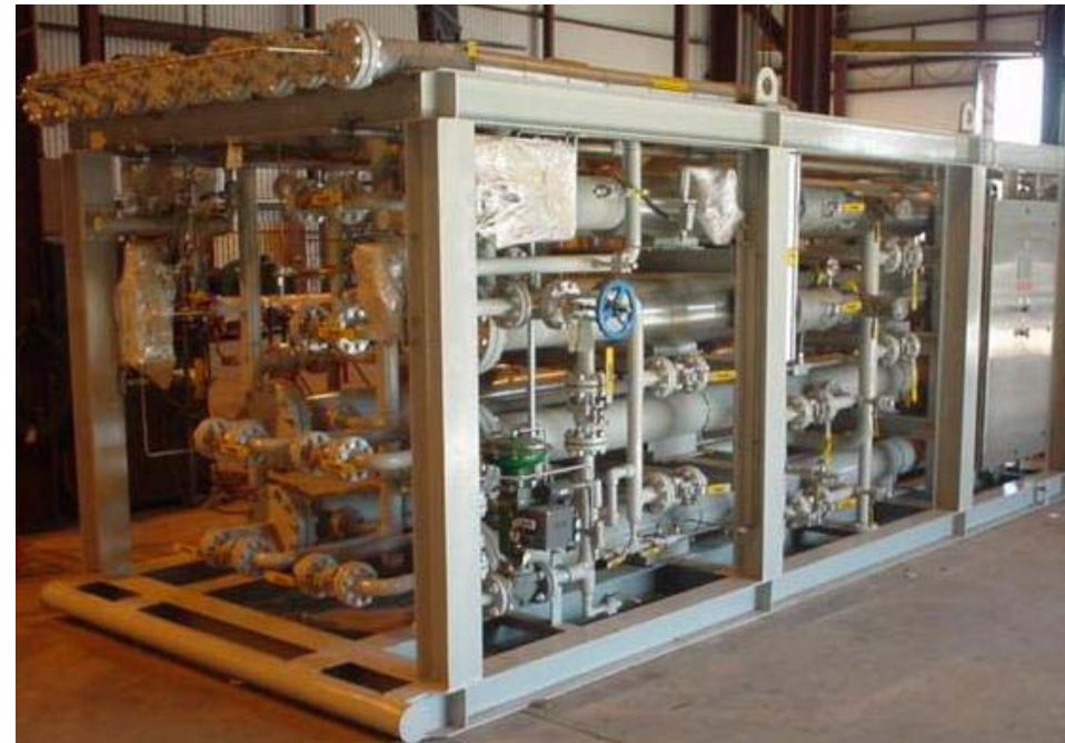
NTE Membrane System Design Flow Rate-1.0 MMSCFD
